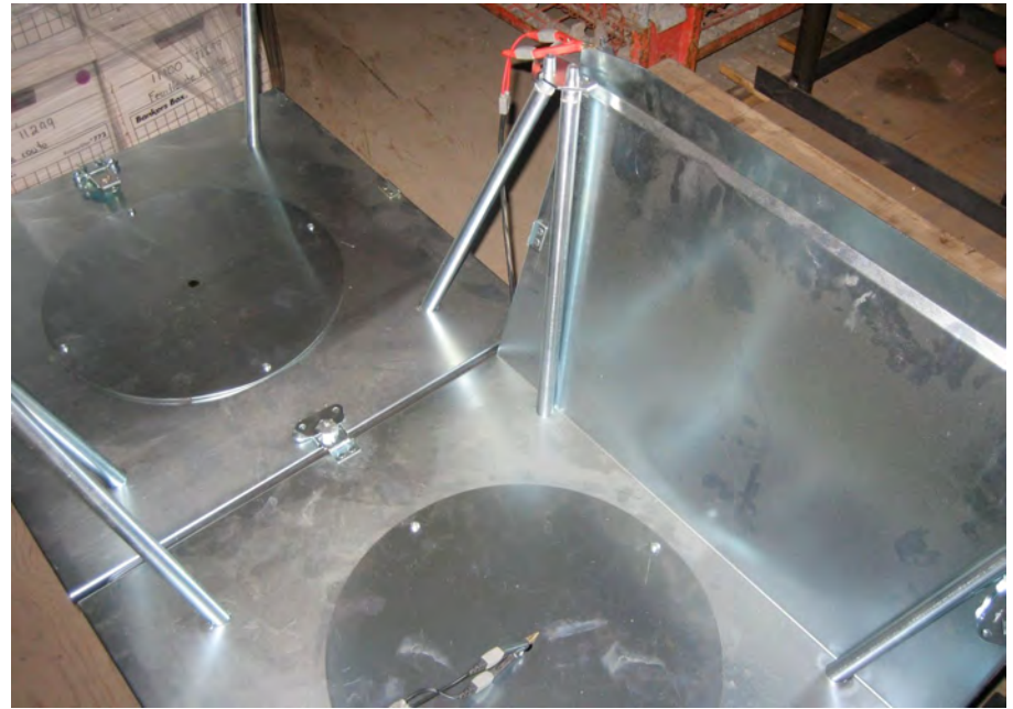
Pic. 3- Center of Module 2 to Top of Outside Perimeter-Reading .3 mOhm
