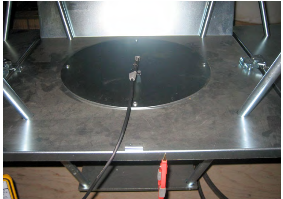
Pic 4- Center of Module 2 to Outer Edge of Pan-Reading .2 mOhm
