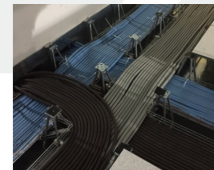
Power cables are simply laid in the upper utility plenum—install 232 cabinets in 1 day
